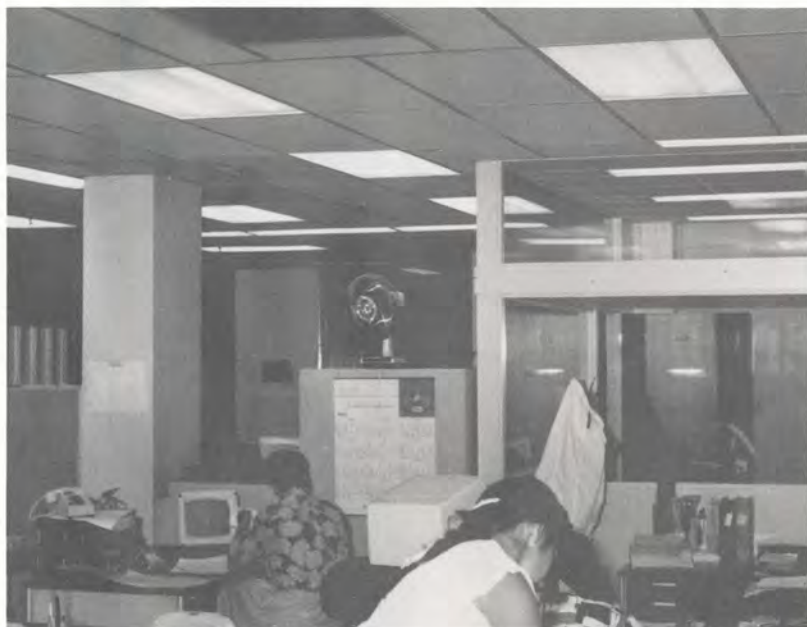
Installed Silverlux reflectors at the Sperling offices create a brighter, softer light.
